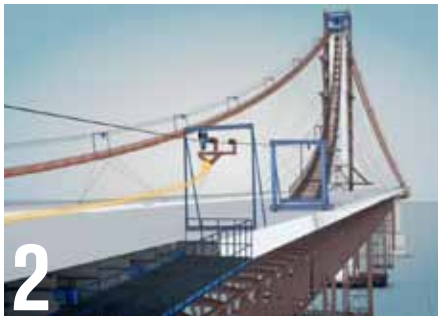
2 Hauling system pulls the strand westbound, the reel remains stationary at the east end of the deck as the strand unspools
